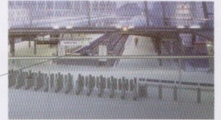
la barrera ticket barrier
